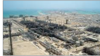
Treatment, liquefaction and export terminal
